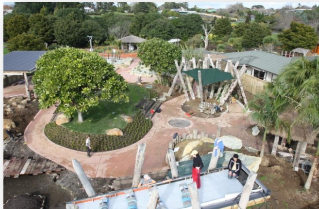
Under construction, the new garden is twice as big as the original
